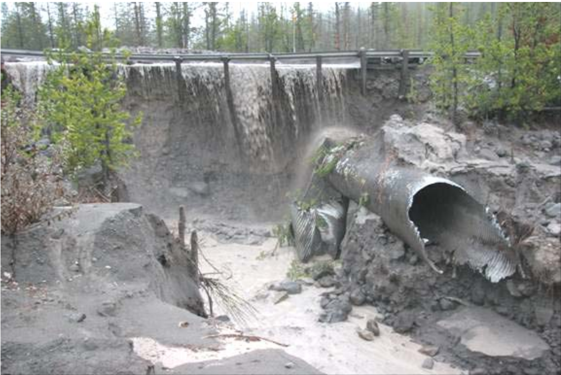
Tributary culvert on the north end of White River bridge. Road 48 is about 50 yds north, to the right. About 2/3 of White River is here.
