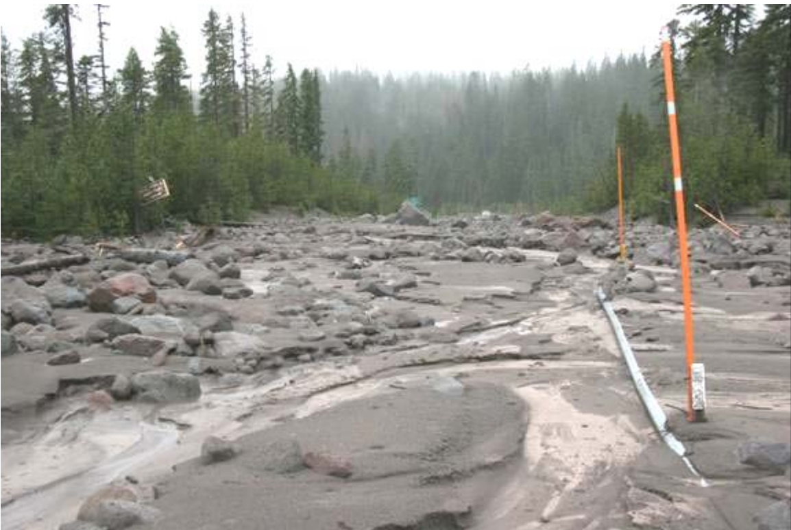
Photo taken from middle of White River bridge looking south. Guardrail and snowpoles mark the upstream side of the bridge! You should be looking down about 15 feet on the right side to where the river is supposed to be.
