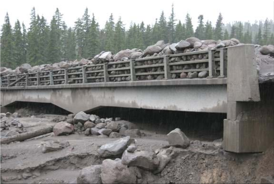
Down River Side of White River Bridge. The top of the pile on the bridge is level with the upstream side of the bridge meaning about 15-20 ft of fill.
