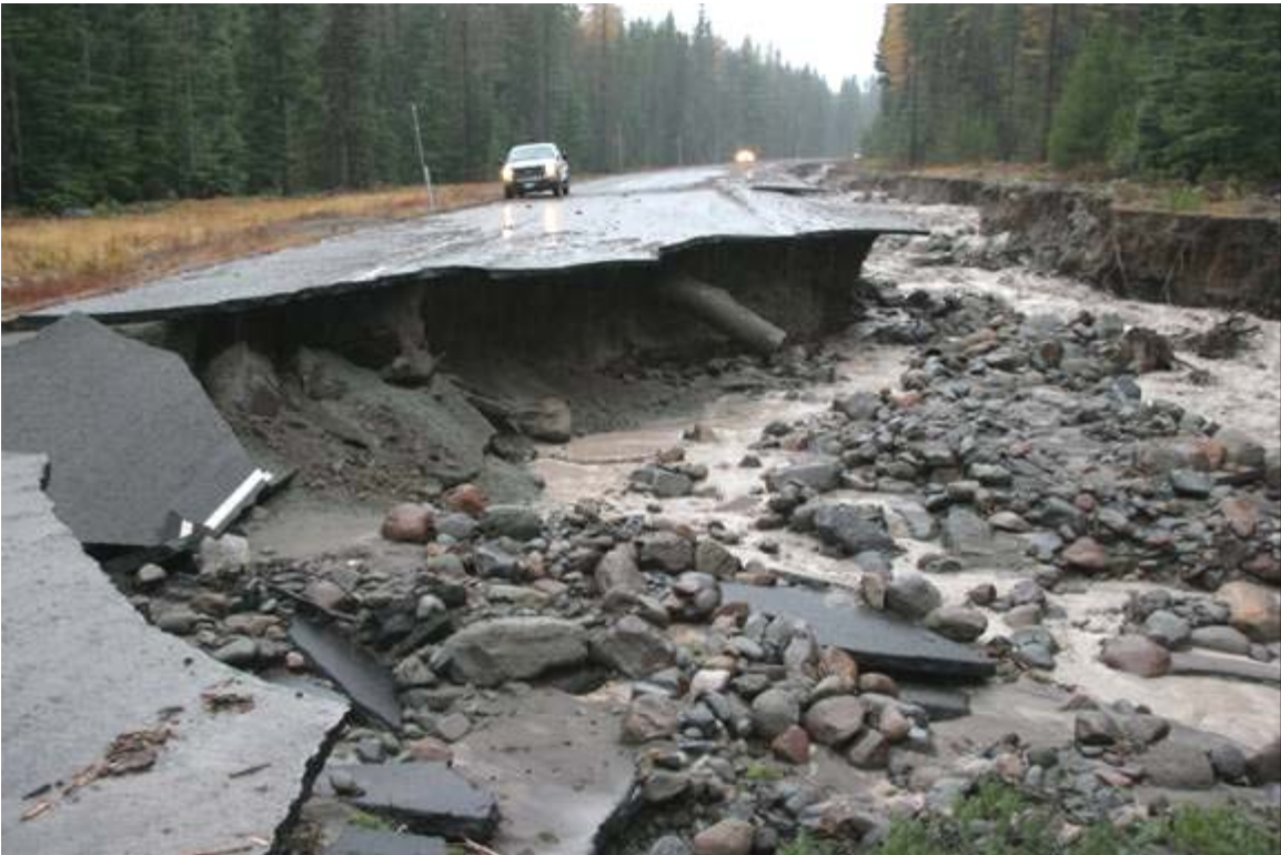
Hwy 35 just south of Pocket Creek snopark. This is Clark Creek flowing along the Westside of the highway toward Newton Creek box culvert where it crosses the road. Newton Creek is now where it was in the last event!
