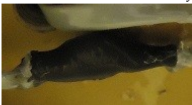
Figure 38: Untwisted Phone Cables
