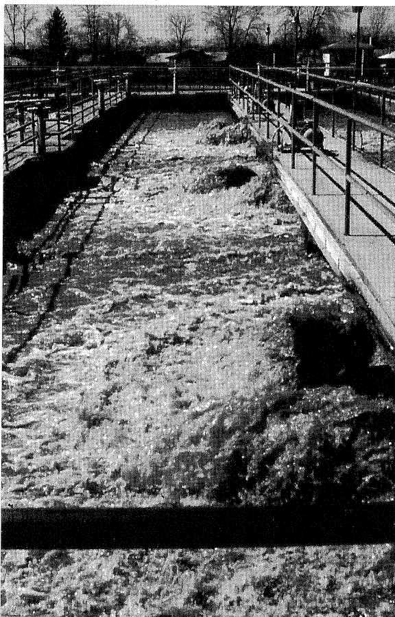
Figure 12.10 Surface aerators in an activated sludge process.
