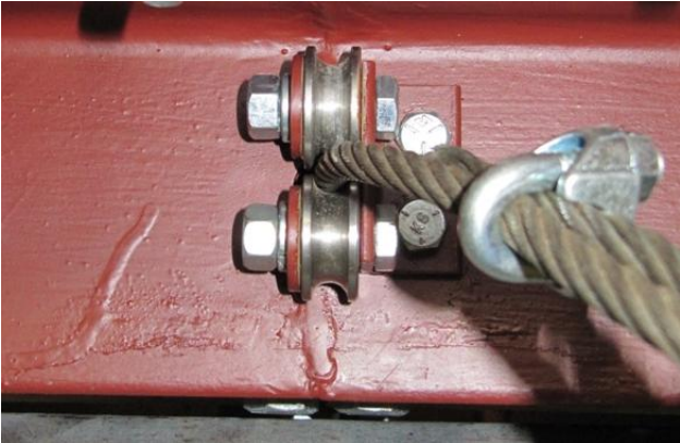
Figure14: Upper cable guide as installed on cart
