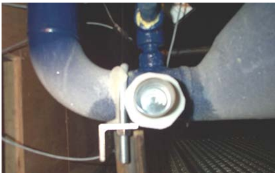
Figure 7-Flow separator entrance sight glass
