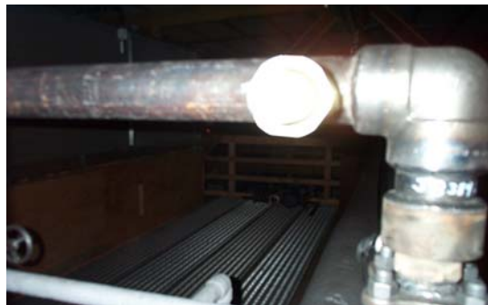
Figure 8-Hot gas supply sight glass
